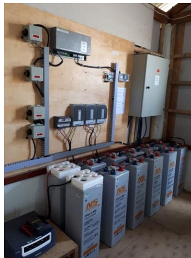
Fig. 9 Battery System for Wind Turbine and PV
