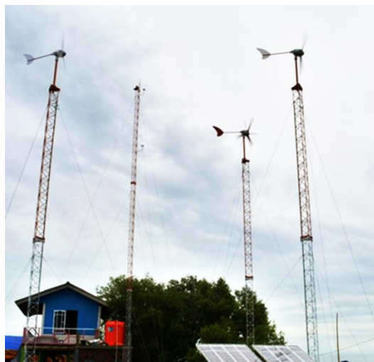
Fig. 5 Installed Wind Turbine and Seawater Desalination
