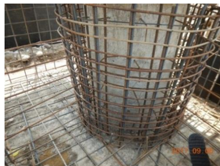
Figure 24. Reinforcement of the Concrete Jacket of the Experimental Model of the Bridge Pier
