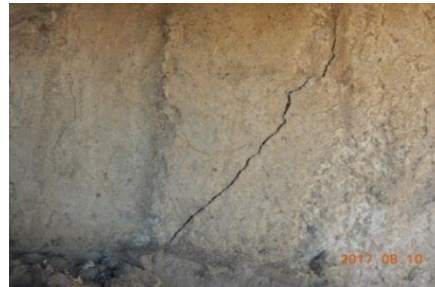
Figure 22. Pier Bridge Shear Crack of the Experimental Model
