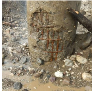
Figure 21. Pier Bridge Corrosion of the Experimental Model
