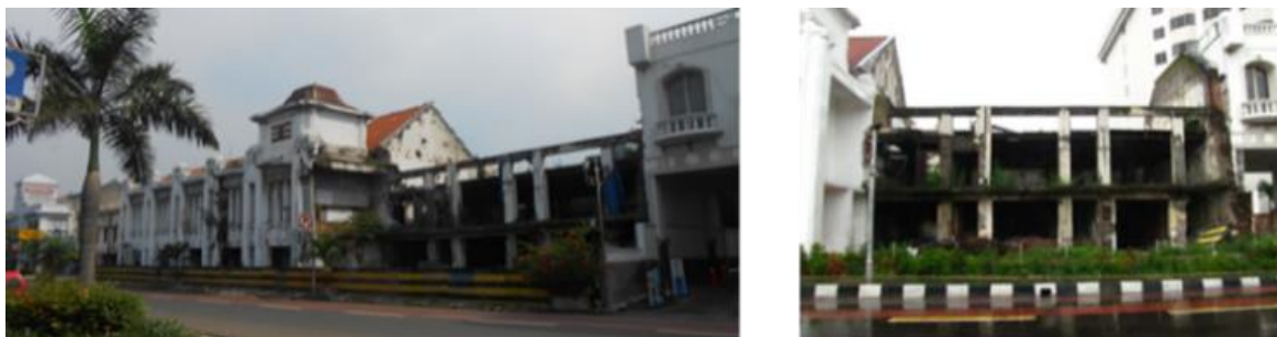
Figure 4. Existing Condition of the Shipping Office Building of Samudera Indonesia Limited, with Half of the Building Destroyed by Land Subsidence
