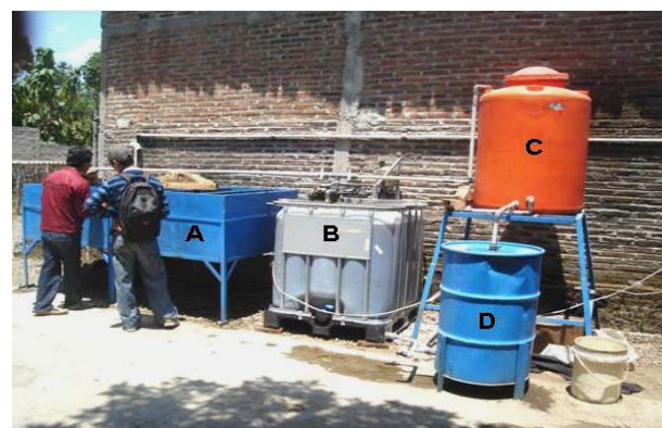
Figure 1. Wastewater Treatment Reactors, i.e. ABR (A), RBC (B), Collecting Tank (C), and Filter (D)
