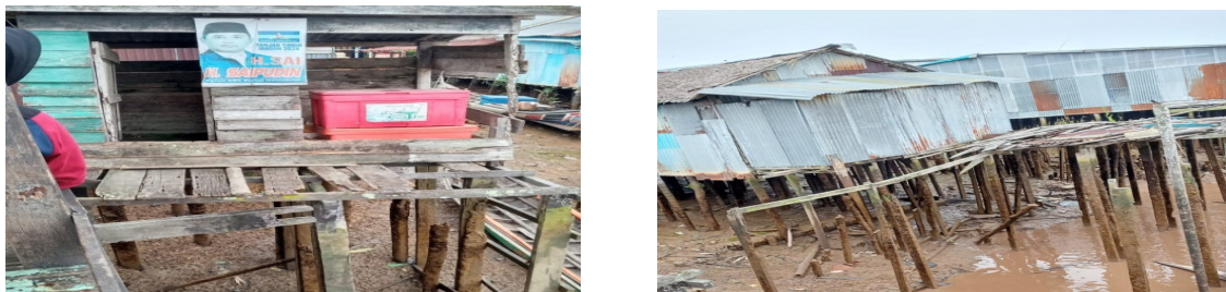
Figure 1. Condition of Family Latrines
