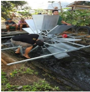
Fig. 1: Community takes part during installation process of pico hydro Source: Dendy Adanta (2017)
