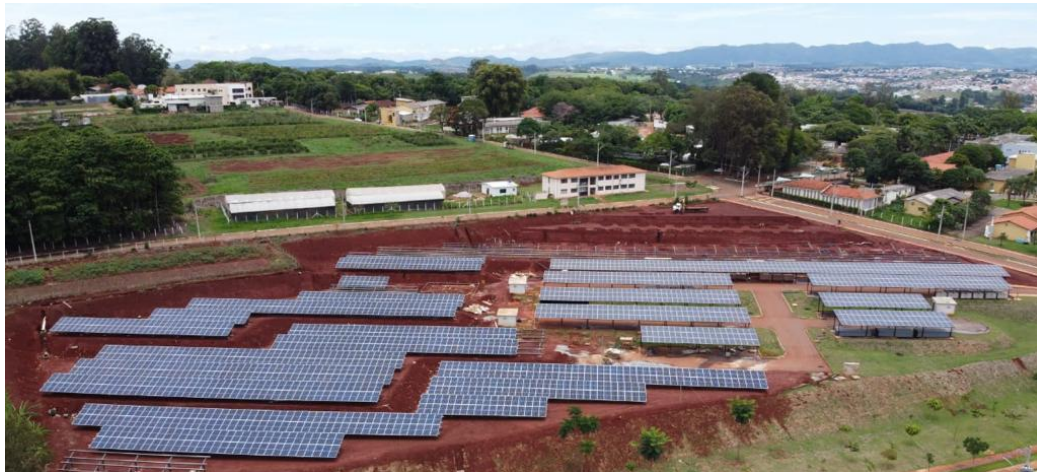
Figure 11. Solar Parking and Solo Plant – 1.263 kW (Source: UFLA, 2016)
