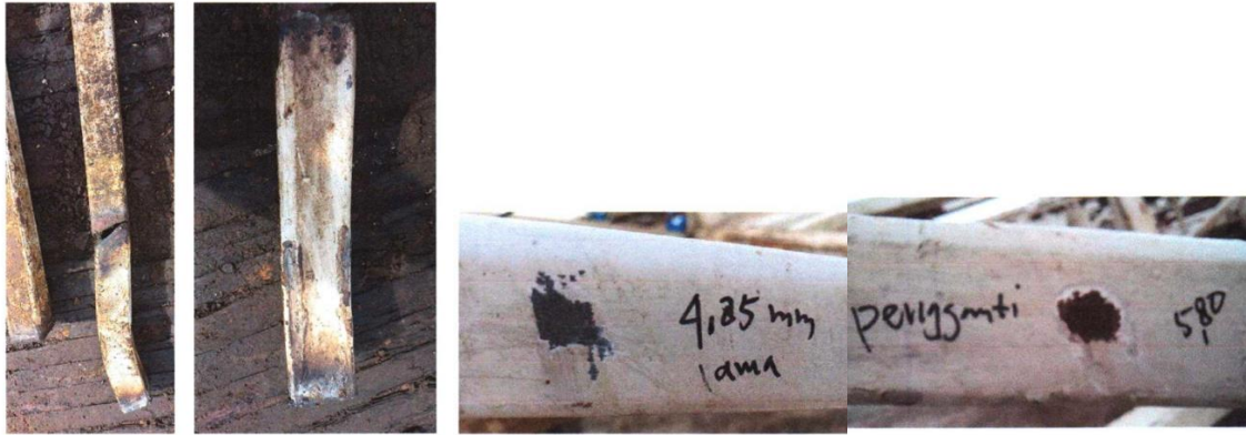
FIGURE 1. Damaged and Replacement Braces
