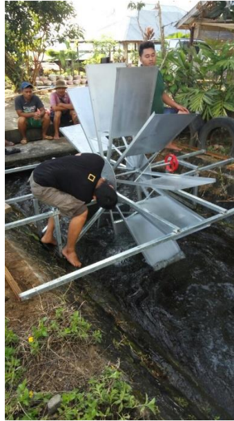
Fig. 3 Community takes part during installation process of pico hydro Source: Dendy Adanta (2017)
